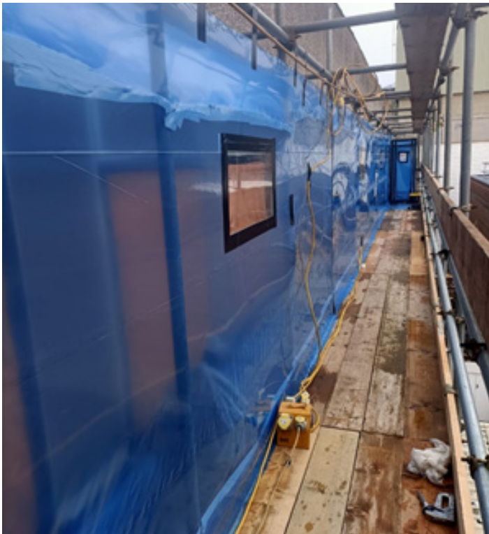
External enclosures accessed via scaffold walkways
